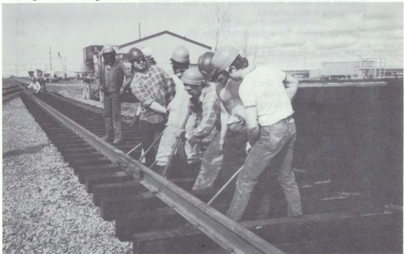
Relaid and turned rail received emphasis during the summer construction season. Here maintenance-of-way employees install new ties, ballast and 78 foot rails at Anchorage Depot.
