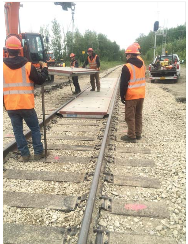
Concrete panels are placed at the crossing with Fairview Loop Road as part of an upgrade in 2014-2015.
