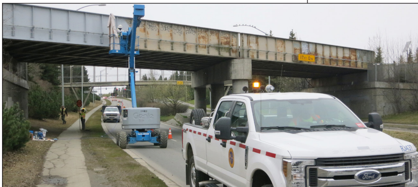
Graffiti clean-up on the rail bridge over Anchorage's Northern Lights Boulevard involves safety measures and lane closures over three days in early May 2018.
