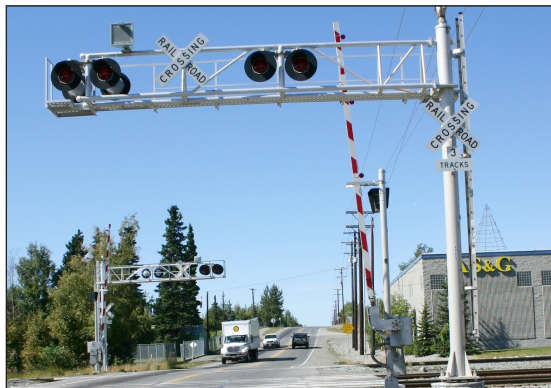
Automated wayside horns at Klatt Road crossing.
