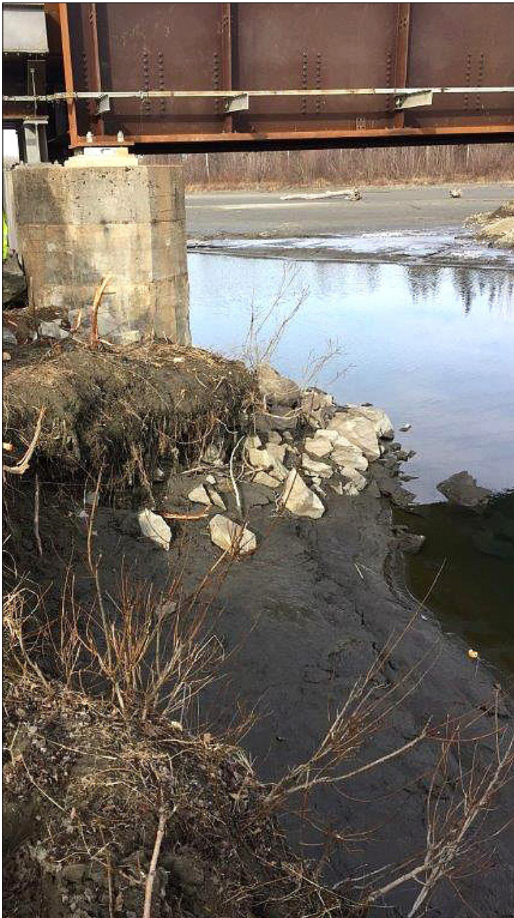
The 2018 earthquake caused settlement and sluffing of track embankment adjacent to the Knik River, near the railroad bridge at MP 147.5.
