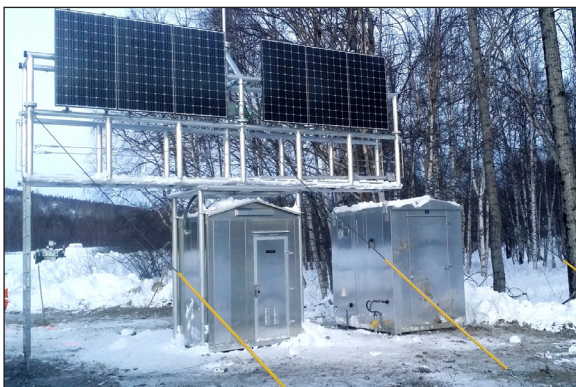
Wayside equipment at Curry is housed in shelters and powered by solar and solid oxide fuel cell technology.
