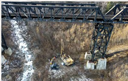
Geotechnical work is completed on the tri-span pony truss bridge at MP 351.4. Performed in 2021, the work supports the capital project to replace the bridge.
