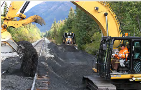
About $20 million of the railroad's 2021 capital budget supported track rehabilitation and repair work.
