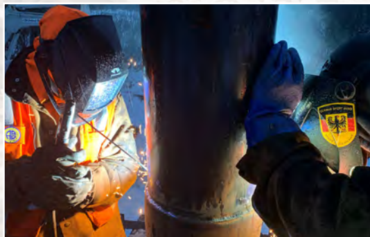
During 2021, members of an Alaska Railroad bridge gang weld steel components on a replacement bridge at MP F9.4 along the Whittier Branch line.
