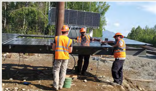
A crew assembles a solar power array at Gold Creek as part of a multi-year project to upgrade solar power at 18 signal waysides. The project was wrapping up in 2021.
