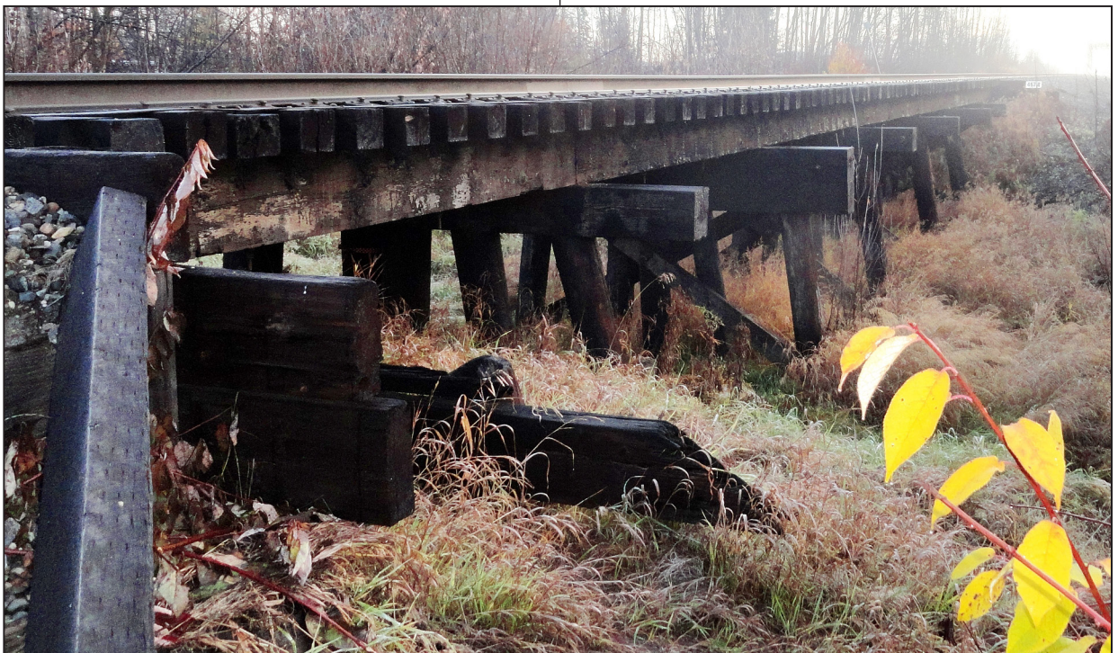
Bridge 467.8 crosses an unnamed drainage flow just south of the Fairbanks Rail Yard.
