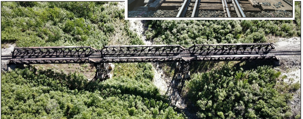
Bridge 351.4 crosses an unnamed gully and creek just north of the Denali National Park entrance.
