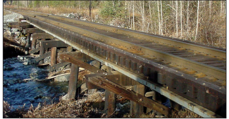
Above: The timber trestle bridge at MP 25.4 over Falls Creek is being replaced with a four-span concrete ballast deck bridge (see drawing at left for reference).
