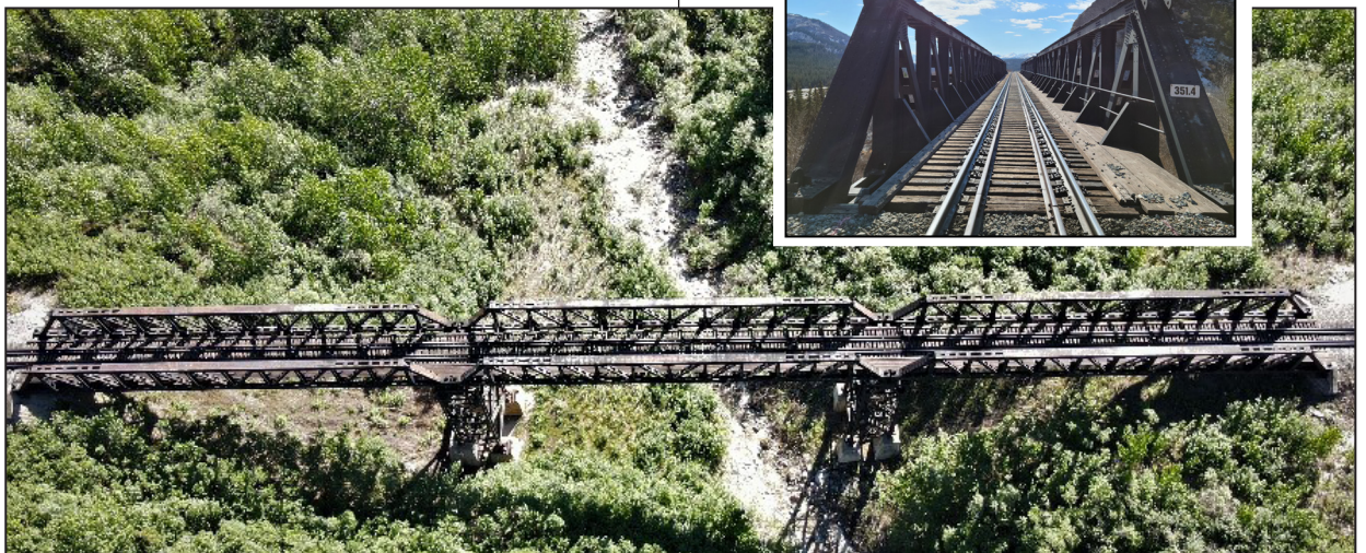
Above: The triple-span pony truss bridge at MP 351.4 will be replaced with a triple-span deck plate girder bridge. Inset: South view of bridge deck at MP 351.4.
