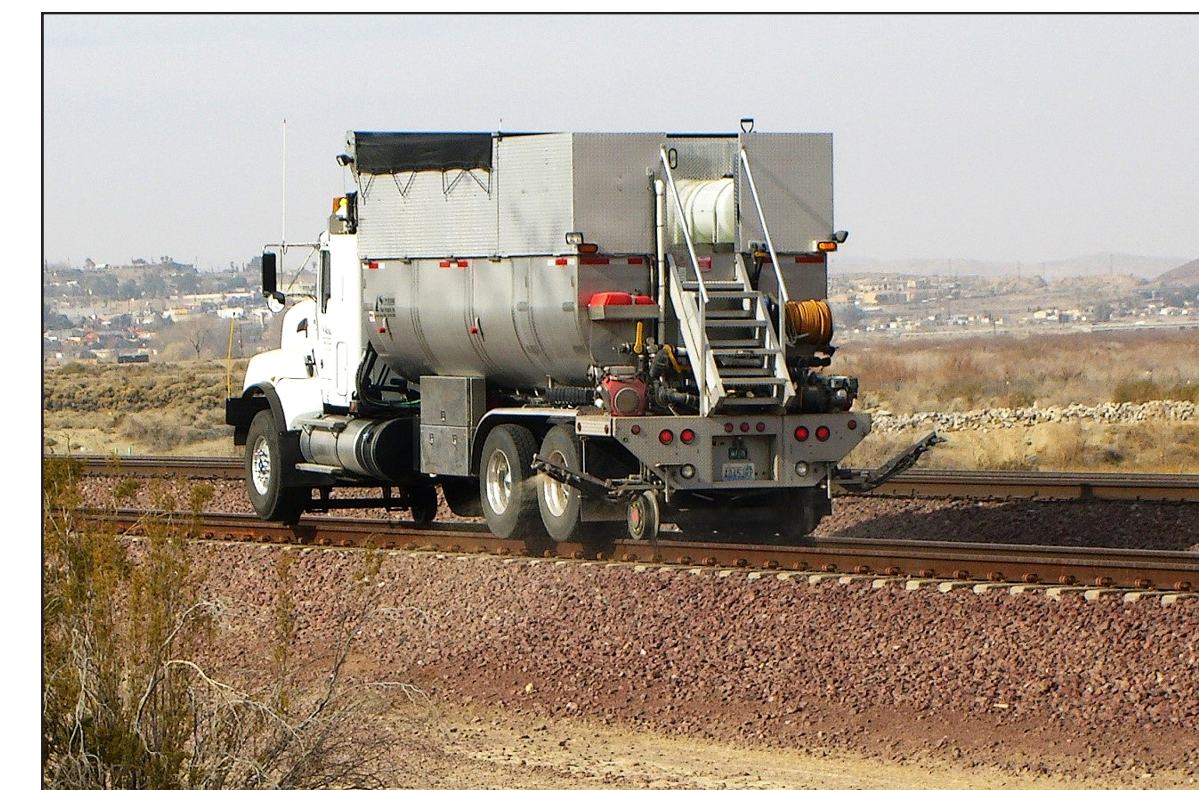
Ferrosafe's specialized hy-rail equipment moves along railroad track to ensure herbicides are evenly directed to avoid trackbed deterioration due to vegetation.
