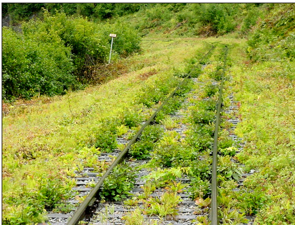
Overgrown weeds on the track are nearly impossible to eliminate with non-chemical methods.
