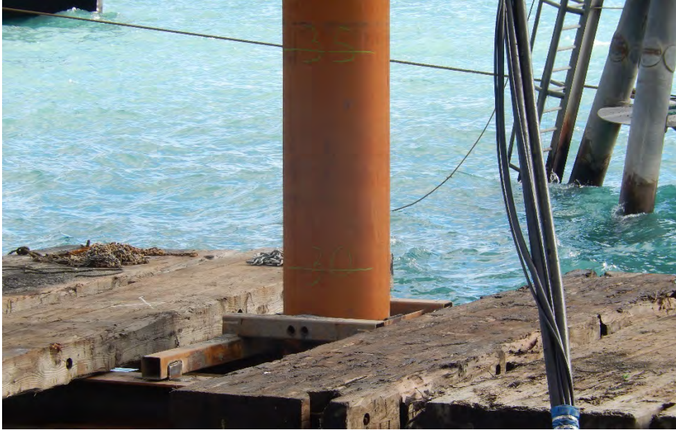
Figure 7 A Steel Pile Set on Location with a Steel Template and Timber Dunnage
