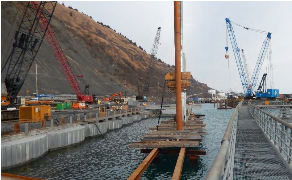
Figure 8 A Pile Being Driven with a Vibratory Hammer and Crane. Note the Template and Land-Based Construction.
