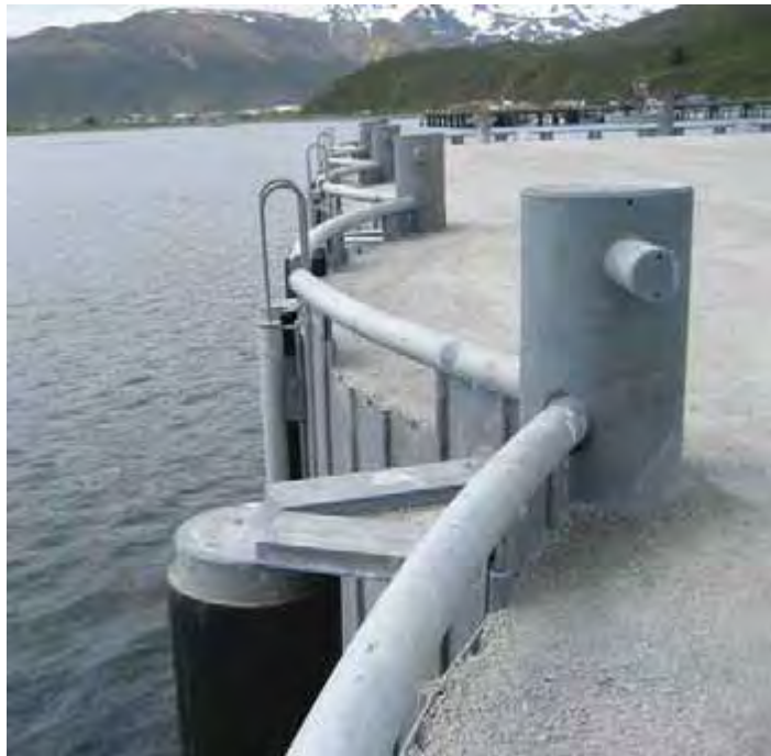
Figure 5 OPEN CELL Dock face with completed Bullrail, Bollards, Fenders, Safety Ladders and Gravel Surface
