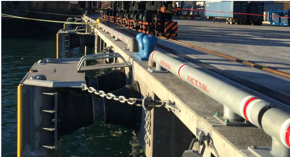
Figure 10 Pile-Supported Dock Face with Completed Bullrail, Bollards, Fenders, Safety Ladders, and Concrete Surface
