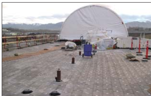
Right: A tent covers the roof area where old utility equipment is removed. Above: A new paved-system roof is installed along with more insulation for energy conservation.
