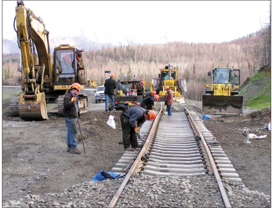
An Alaska Railroad crew installs new track that is improved with continuously welded rail and concrete ties.
