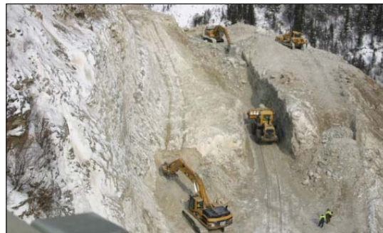
Crews clear debris after a demolition explosion April 17, 2008. Tunnel daylighting was completed in 2009.
