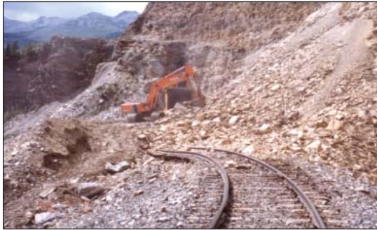
1999: A rock slide at Garner Tunnel closed the track for 24 hours. No one was injured.
