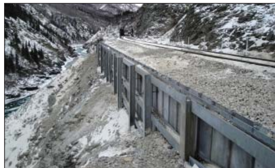
The track retaining wall at MP 354.1 is replaced with a well-engineered improvement.
