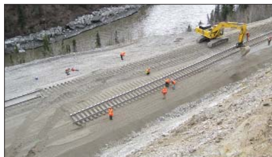
The track at MP 357 is moved further away from the Nenana River with a realignment project during 2011.
