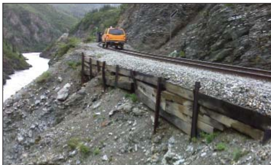
The track bed retaining wall at MP 354.1 needs to be replaced.
