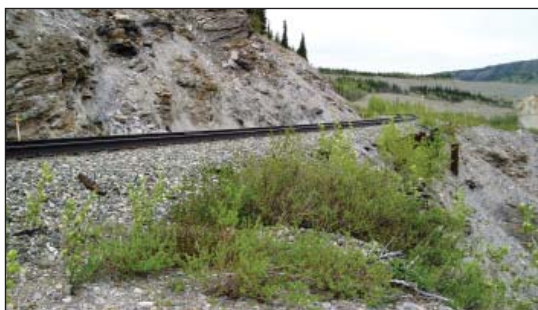
The retaining wall at MP 357 is deteriorating and the track needs to be realigned away from Nenana River.
