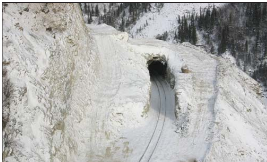
2008: Moody Tunnel is prepped for the demolition step to remove the top from the tunnel.
