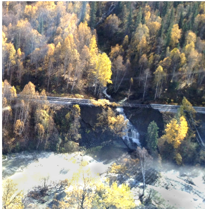
Major washout just south of Gold Creek.
