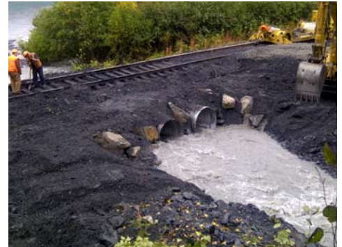
A track washout about 20 miles north of Seward is repaired with newly-installed culverts.
