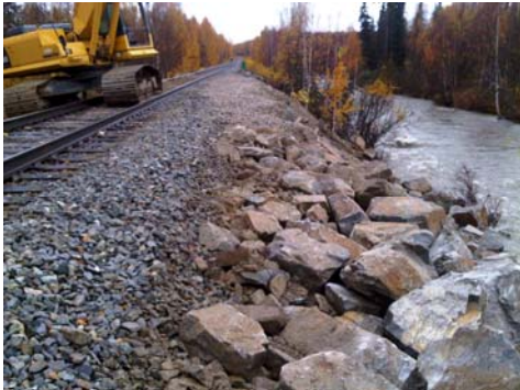
Crews finish placing rip-rap at Sheep Creek to fortify railroad bridge abutment there.
