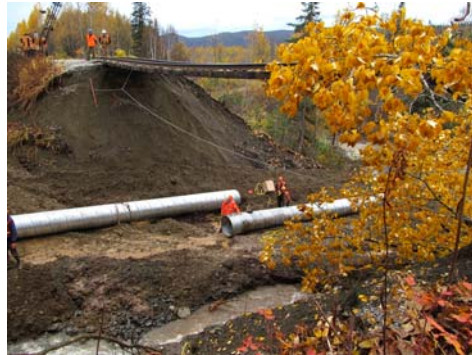
Crews install a culvert under the track at ARRC MP 261 to divert the flood-formed water channel that caused the washout.
