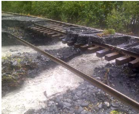
Flooding on the south end of the track causes several small washouts, including this one about 20 miles north of Seward.
