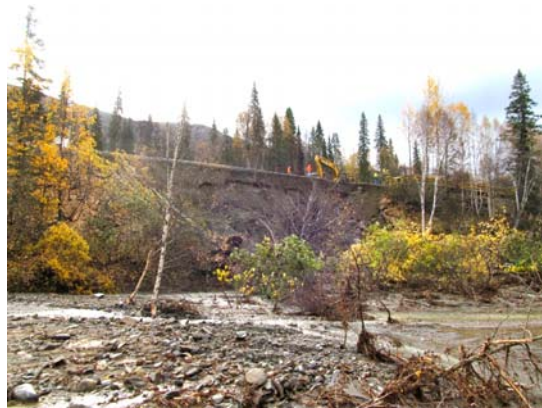
Crews make good progress on the large washout at MP 261, filling the gap with an estimated 20,000 cubic yards of material.
