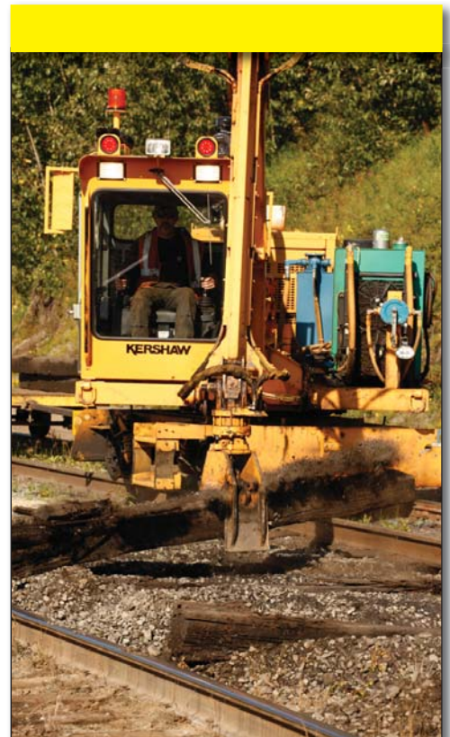
Limited capital funding is focused on critical track repair and rehabilitation work.
