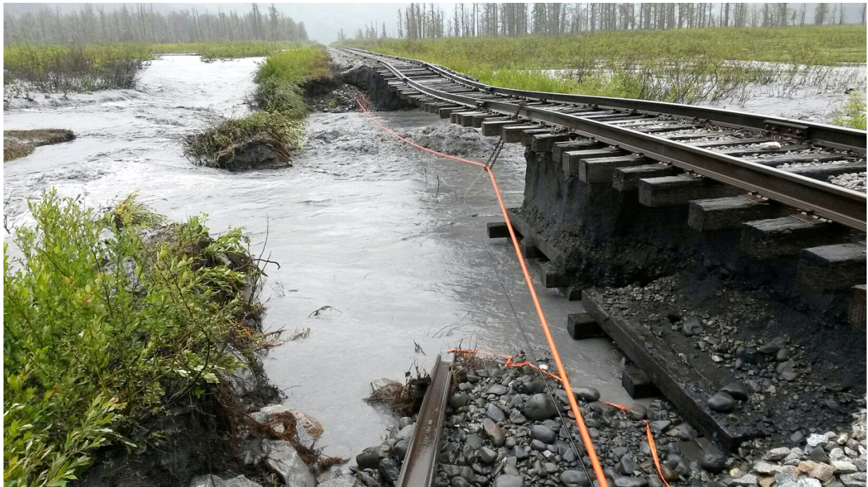
Skookum Creek high water eats away at the trackbed, leaving the tracks suspended.
