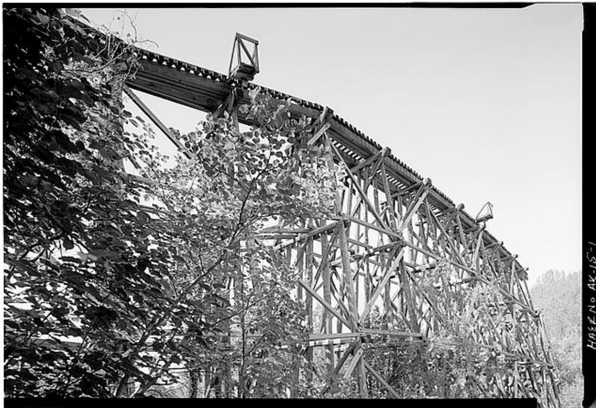
Photograph from the HAER Collection, showing the Copper River & Northwestern Railroad's Gilahina Bridge, timber trestle, built in 1911.
