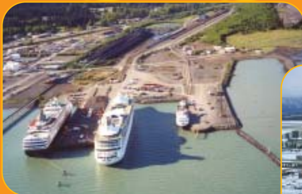
The railroad began renovating the existing Seward general purpose dock into a renovated passenger-only facility.
