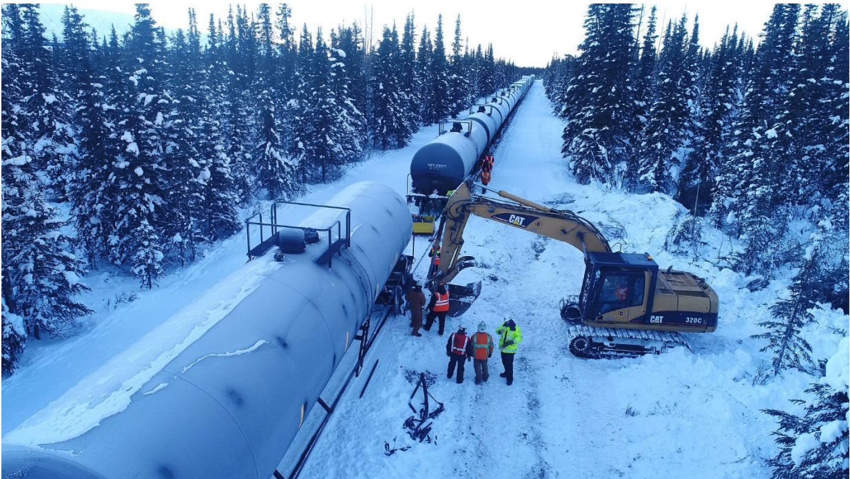
Alaska Railroad heavy equipment is used to help place a derailed tank railcar back on the track.
