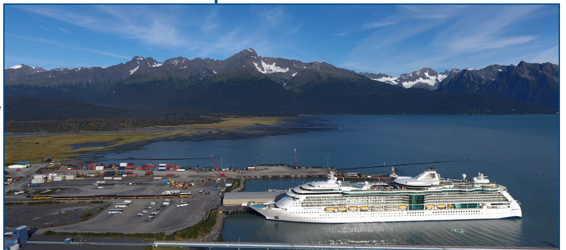
Top: Underside of the Seward passenger dock, photo taken in Sept. 2023, showing significant corrosion and age. Bottom: Seward passenger dock with cruise ship at berth.
