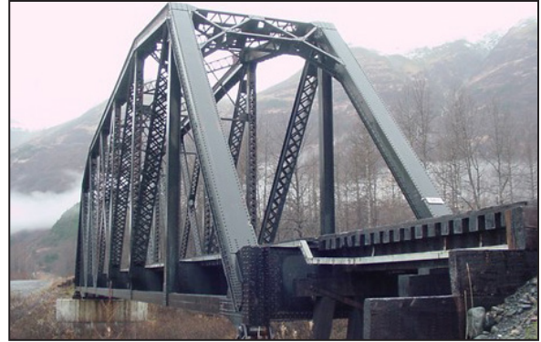
Above: The bridge at MP 54.1 over the Placer River near Spencer Glacier is being rehabilitated, including replacing four (4) 15-foot timber approach spans and abutments with two (2) steel beam spans and abutments.
