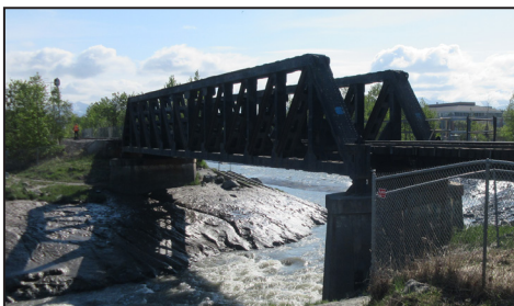
Left: ARRC will replace the 123-foot pony truss bridge crossing the Ship Creek in Anchorage, Alaska (MP 114.3) with two 79-foot beam spans and one 30-foot beam span.
