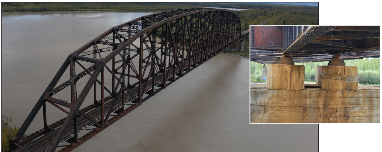
Above: ARRC received an FRA CRISI (Consolidated Rail Infrastructure And Safety Improvements) Program grant to rehabilitate this 1,298-foot, 12-span through truss bridge over the Tanana River in Nenana, Alaska (MP 413.7).
