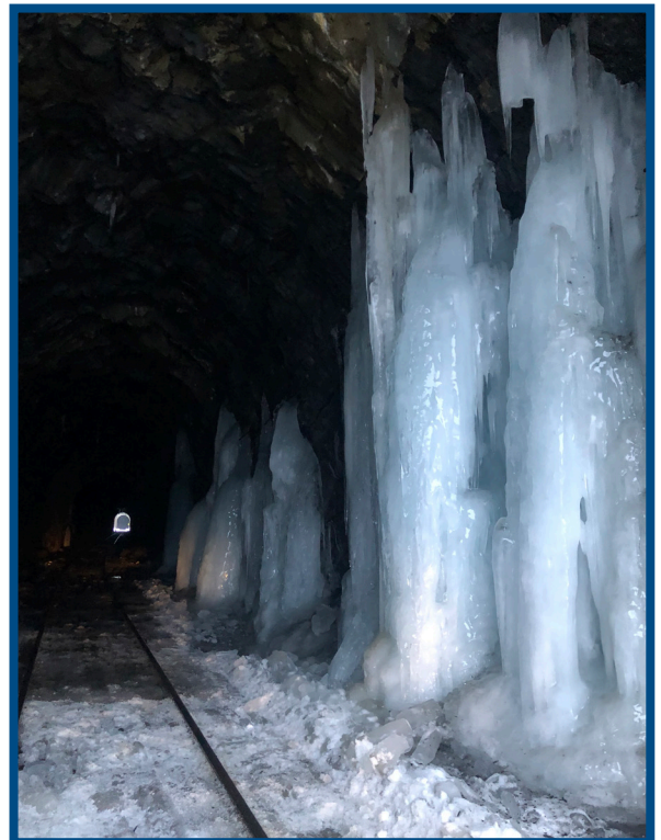
Ice formation inside tunnel.
