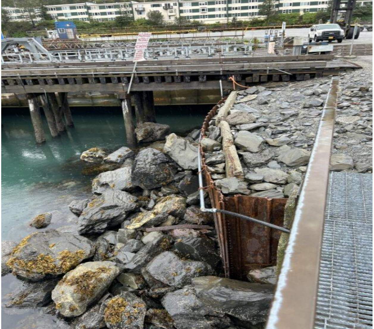
Figure 19. East end of marginal wharf where it connects to barge transfer span.
