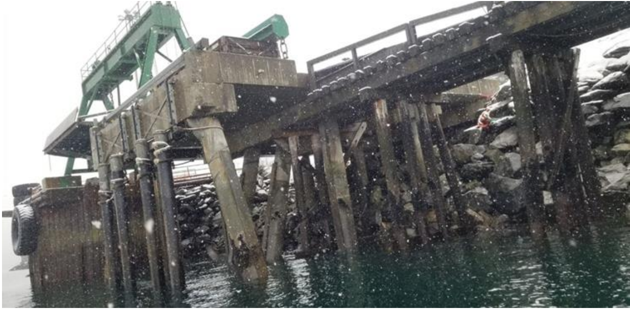
Figure 22. Barge dolphin (left) with fendering and transverse loading ramp within the barge slip.
