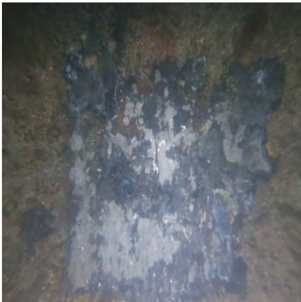
Image 11 – Typical corrosion found
