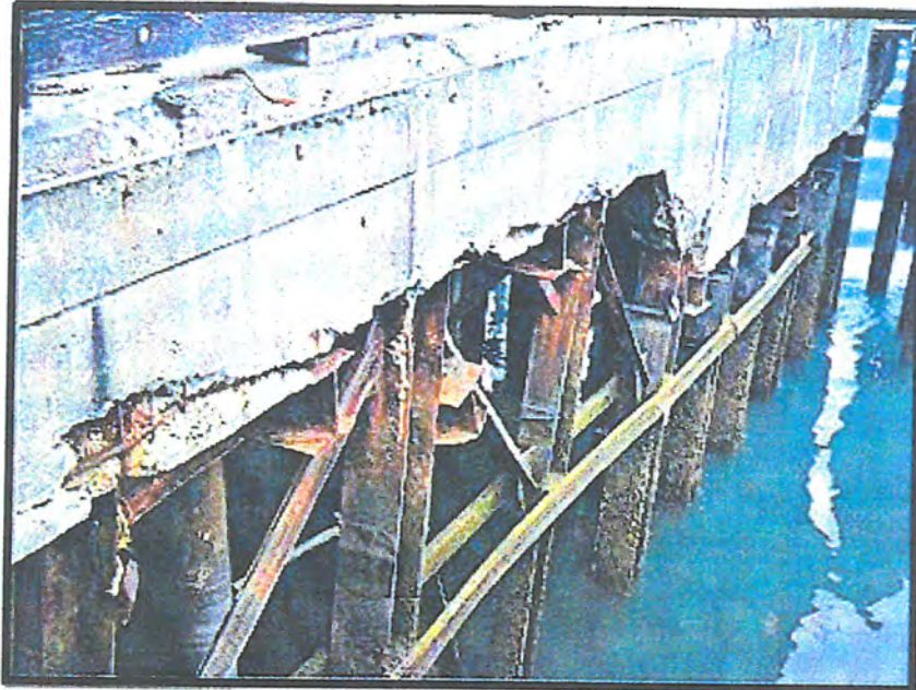
Photo 3: Marginal Wharf: corroded piles and damaged cap
