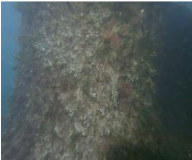
Image 28 – Typical Pile Growth near surface
