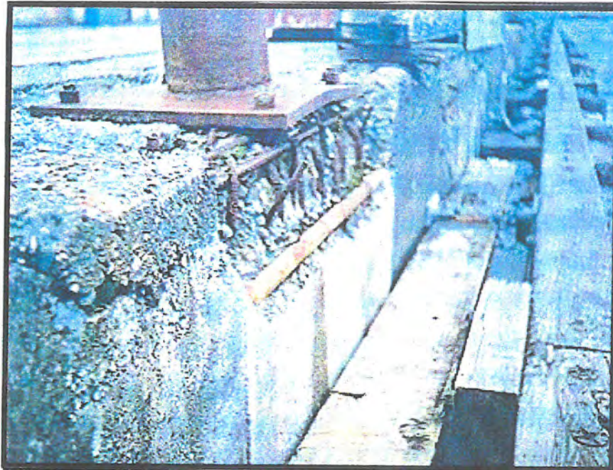
Photo 5: Marginal Wharf: exposed reinforcement in pile cap
