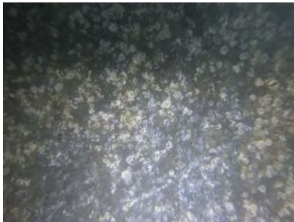
Image 21 – Typical Surface Condition
