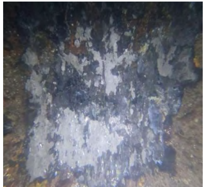
Image 12 – Close up of corrosion
