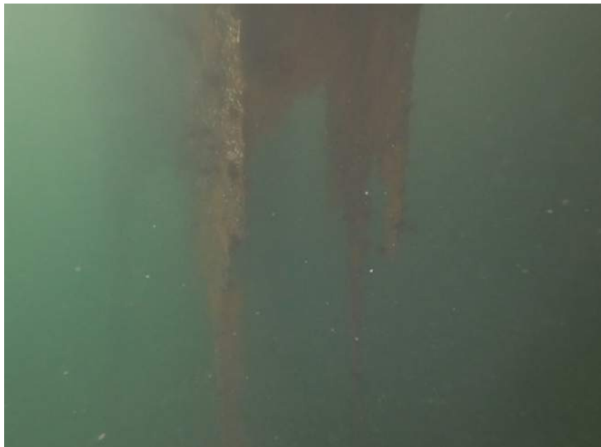
Image 20 – Typical H-Pile Condition at Slip Cells
