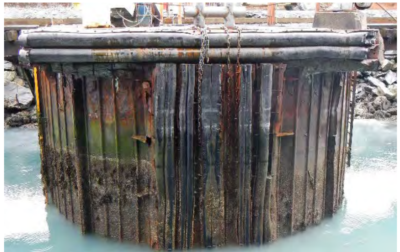
Figure 5 - Sheet piling highly corroded and damaged
