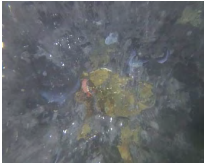
Image 15 - Close up of pitting and corrosion
