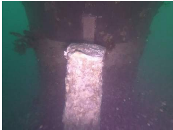
Image 22 – 2020 installed anode typical
