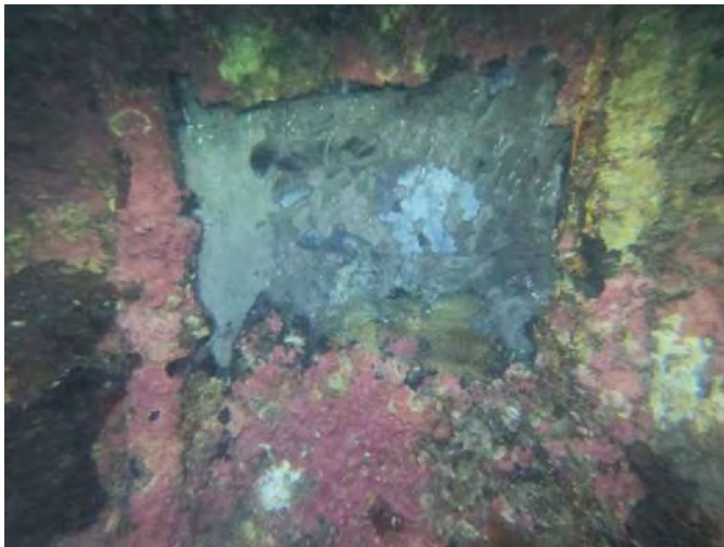
Image 16- Heavy corrosion, pitting and material loss
