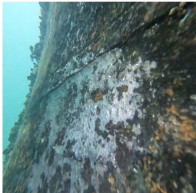
Image 7 – Knife Edge Corrosion Pile Weld
